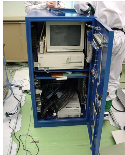
Sealed box including data collection computer
