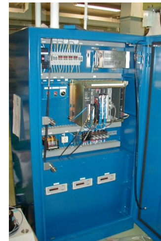
Sealed box including transformer of pressure to electric signal
